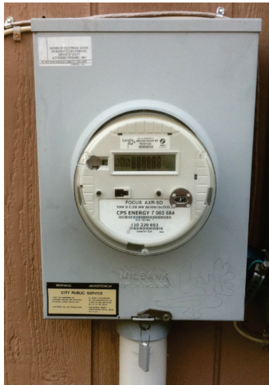
Figure B-1 Landis+Gyr Gridstream smart meter utilized in the test, as installed in the CPS energy residential pilot project.
